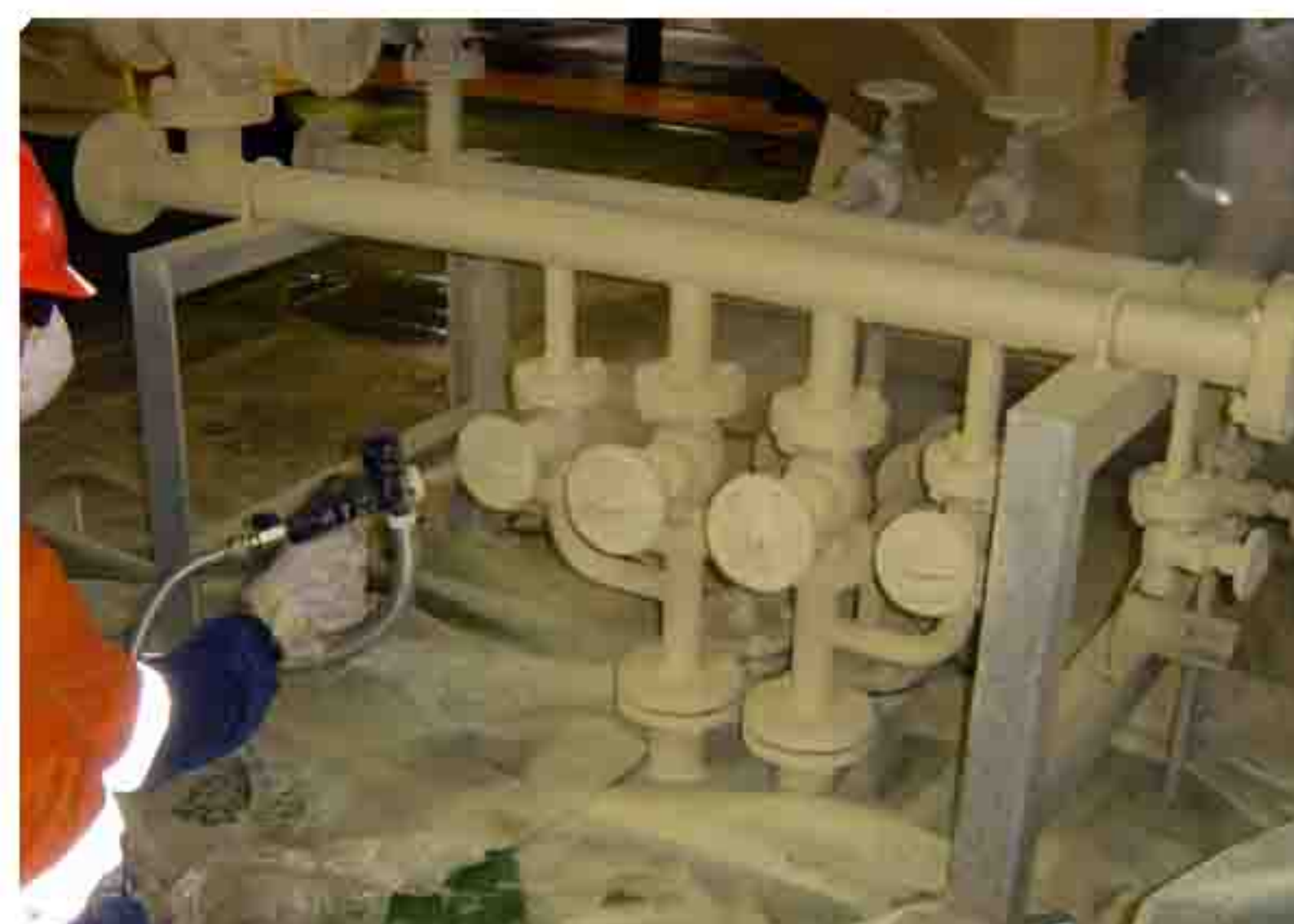
Off-shore application - after
