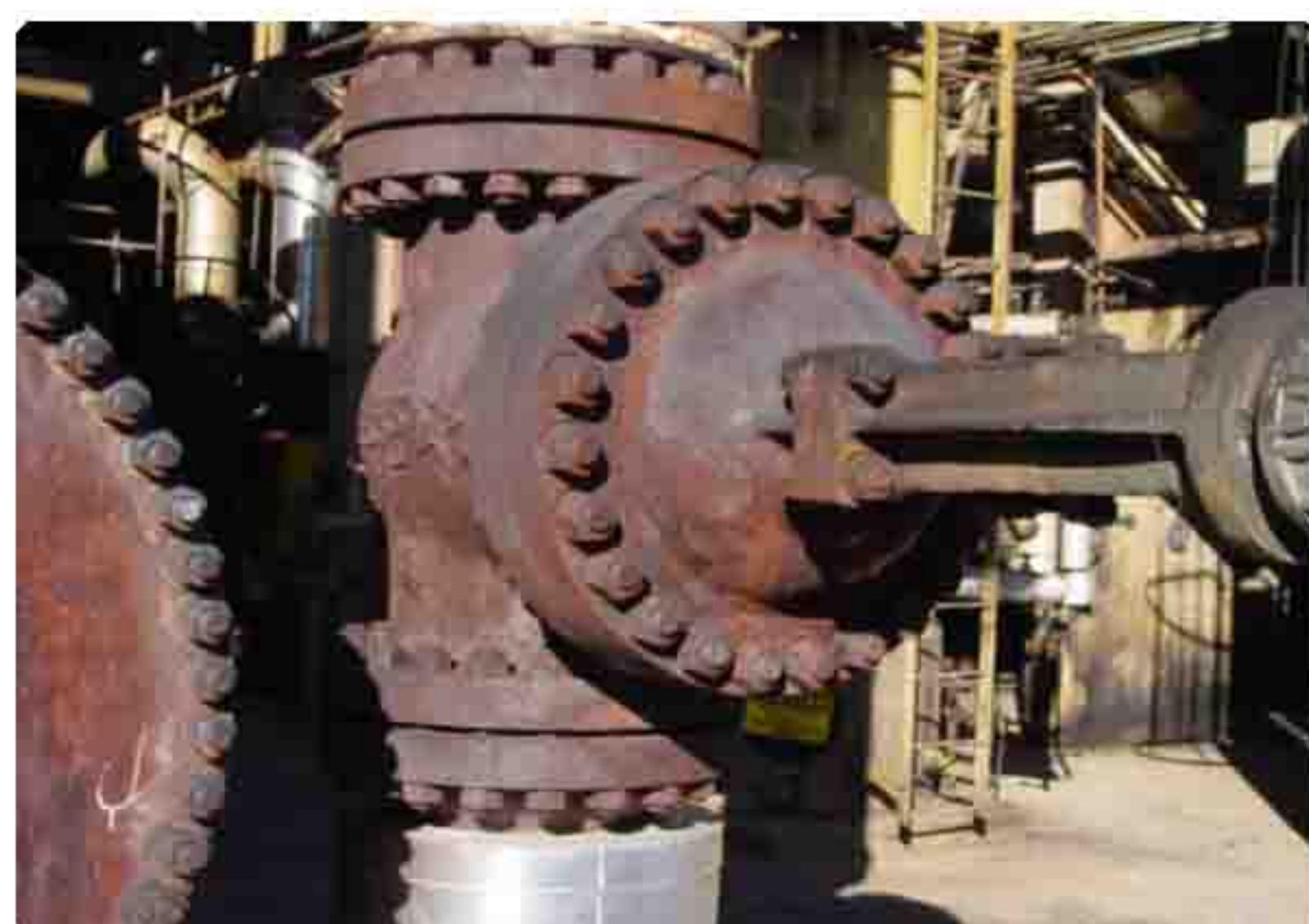
Steam Pipes - [before]
