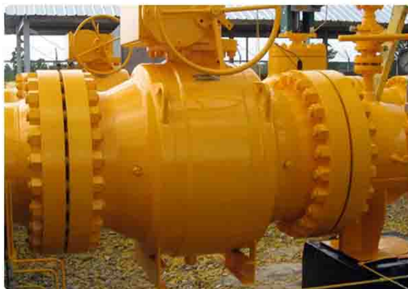
Gas Pipeline - Indonesia
