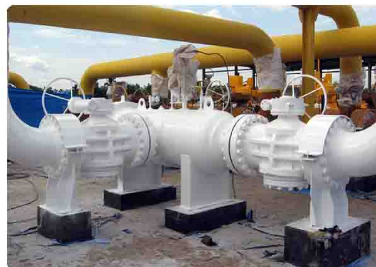
Gas Pipeline - Indonesia
