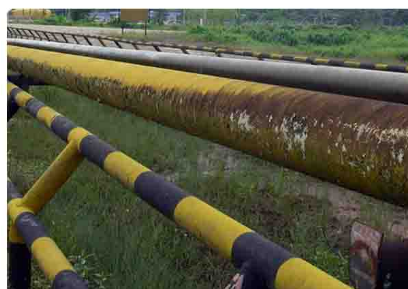
Gas Pipeline - Indonesia
