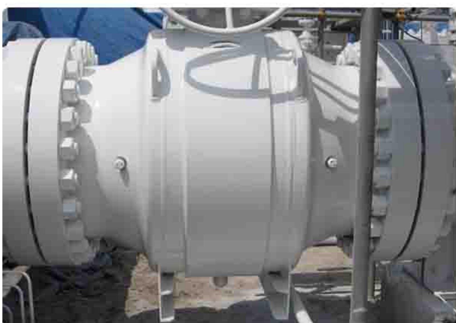
Gas Pipeline - Indonesia
